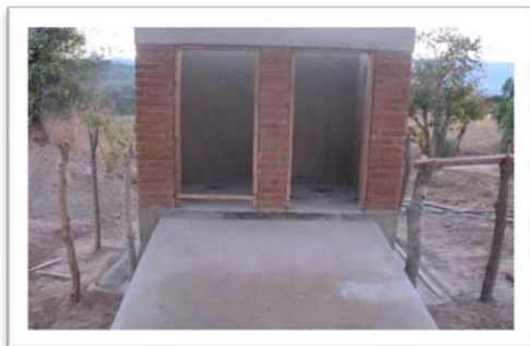
Figure 4: Ramps in school toilets in Malawi enable access for pupils with a disability. Photo: WaterAid
